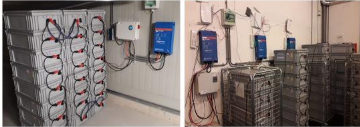
back up energy storage
