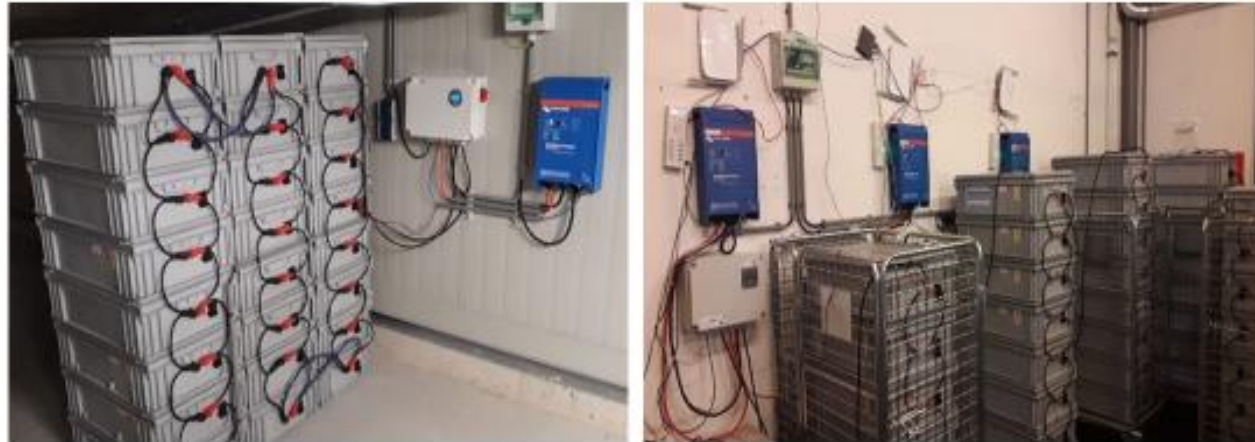
back up energy storage
